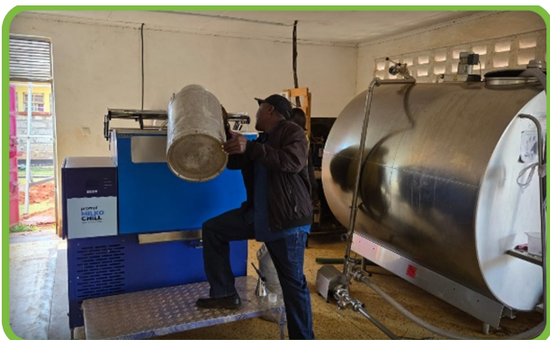
Milk-O-Chill solution being installed and tested at a site in Kenya
